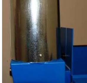
Figure 11. Secure Exhaust Ventilation Stack
