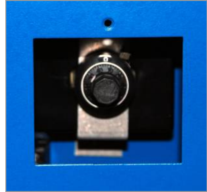
Figure 25. Blower Speed Control (Close Up)
